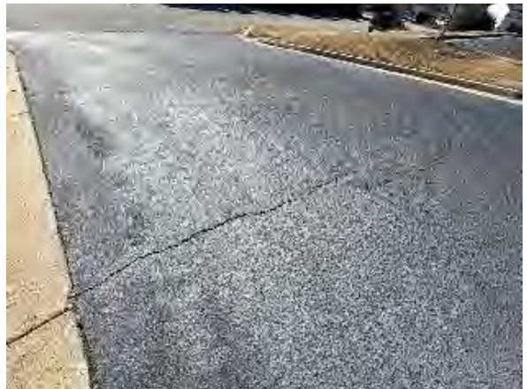
Parking Lot - Cracking
